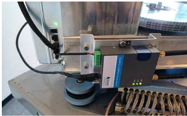
Figure 2-33: LTE modem connection, example
